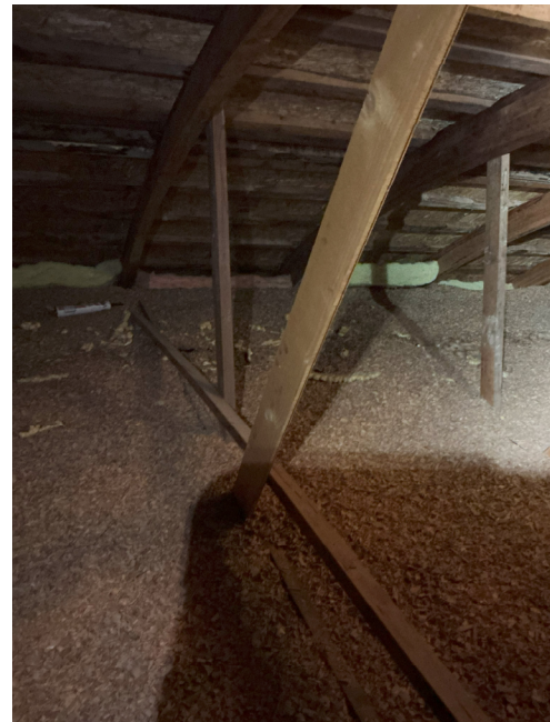
Photograph 5: Broken arch & ceiling support (lower horizontal piece is broken off arch)
