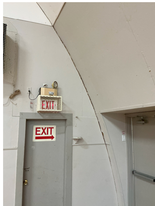
Photograph 10: Displacement at southwest corner
