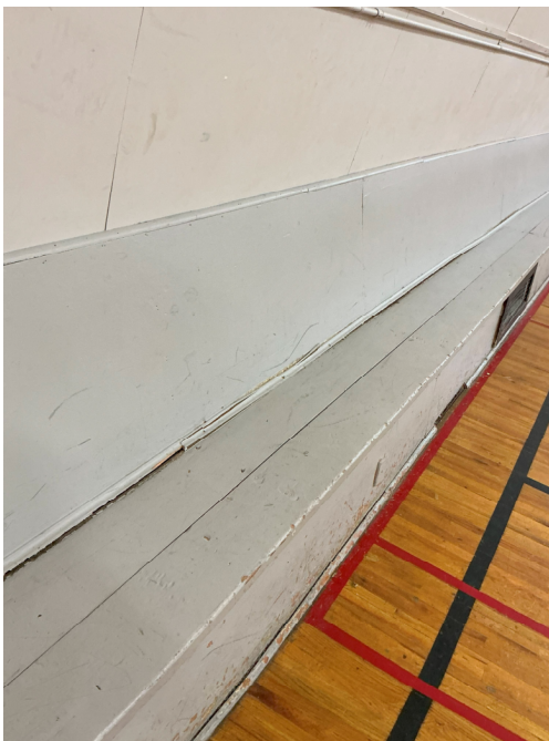
Photograph 9: Splitting / displacement at back of bench
