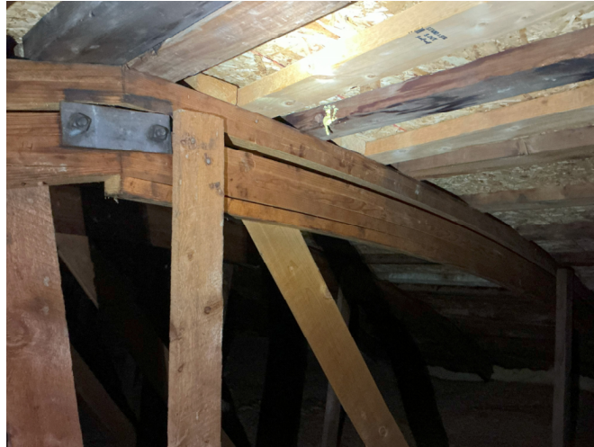
Photograph 6: Broken / delaminated arch at peak connection
