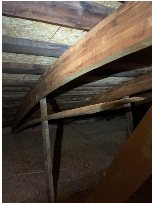
Photograph 4: Broken glulam arch
