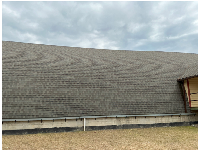
Photograph 7: Bulging / alteration of roof along central portion of west side
