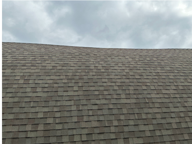
Photograph 8: Bulging / alteration of roof along central portion of west side
