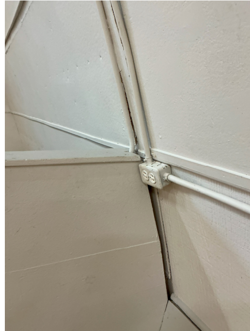
Photograph 12: Wall displacement away from conduit
