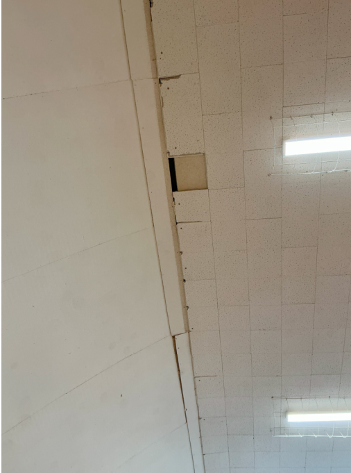
Photograph 11: Finishes pulling apart at ceiling
